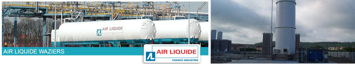
Figure 3. Horizontal and vertical liquid hydrogen storages. (Source Air Liquide).
